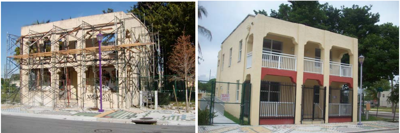
The structure of the Ward Rooming House had to be stabilized (left). The picture to the right shows the restored Ward Rooming House.
