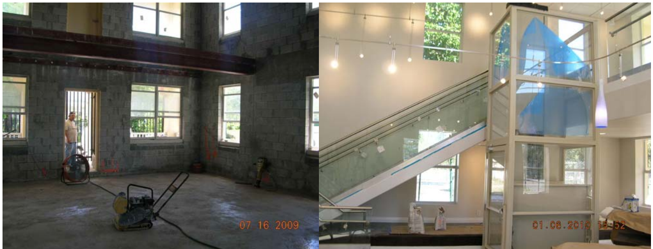
The interior of Ward Rooming House during construction (left). The picture to the right shows the interior built out.
