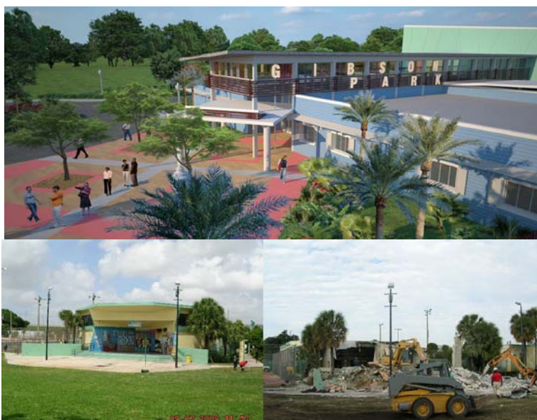
Construction is underway at the Gibson Park site at 401 NW12 th Street, in Overtown.
