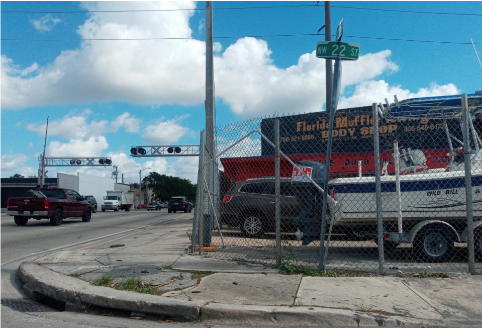
Exhibit: This photographic evidence shows unsafe conditions (cracked sidewalks) for pedestrian and people with disabilities.
