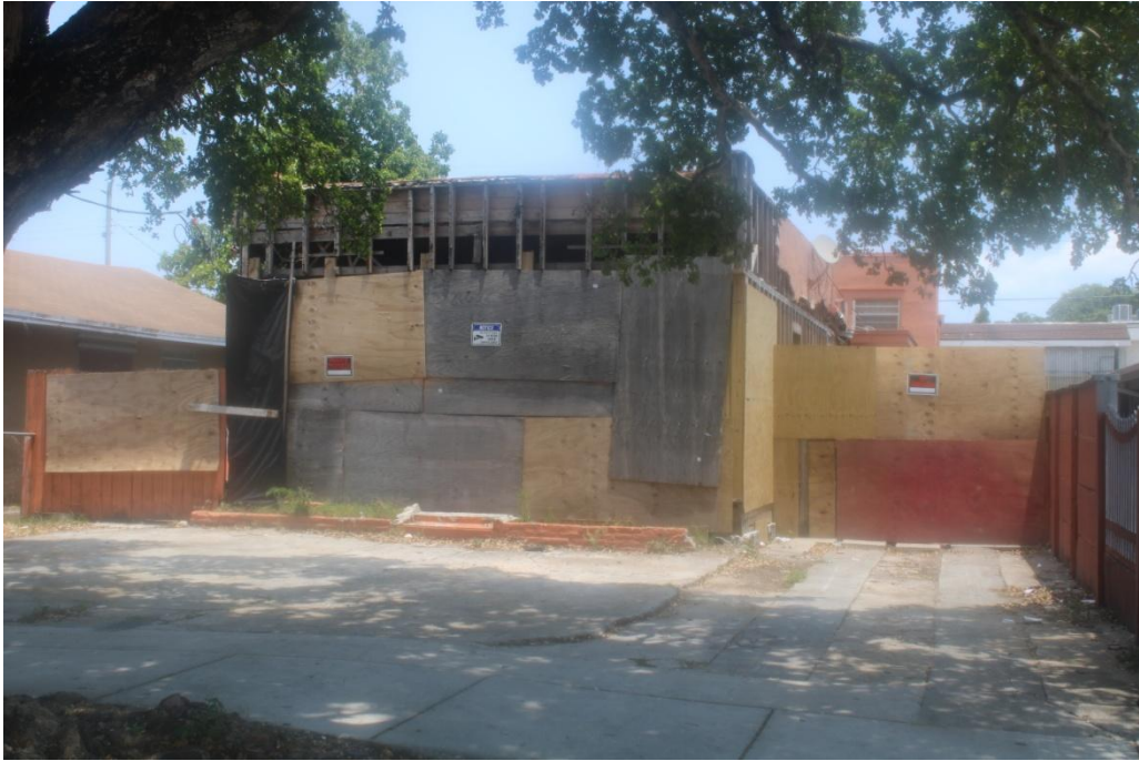
Exhibit: This photographic evidence shows signs of building deterioration. In addition, the basic infrastructure of curbs, sidewalks and streets throughout the Study Area is in poor condition or in disrepair, and fail to meet current American with Disabilities Act (“ADA”) standards. Multi-family residential buildings exhibit deteriorating conditions resulting from long-term neglect. Some buildings have been demolished because they were deemed unsafe, and in turn, the number of vacant, unimproved properties in the Study Area has increased.
