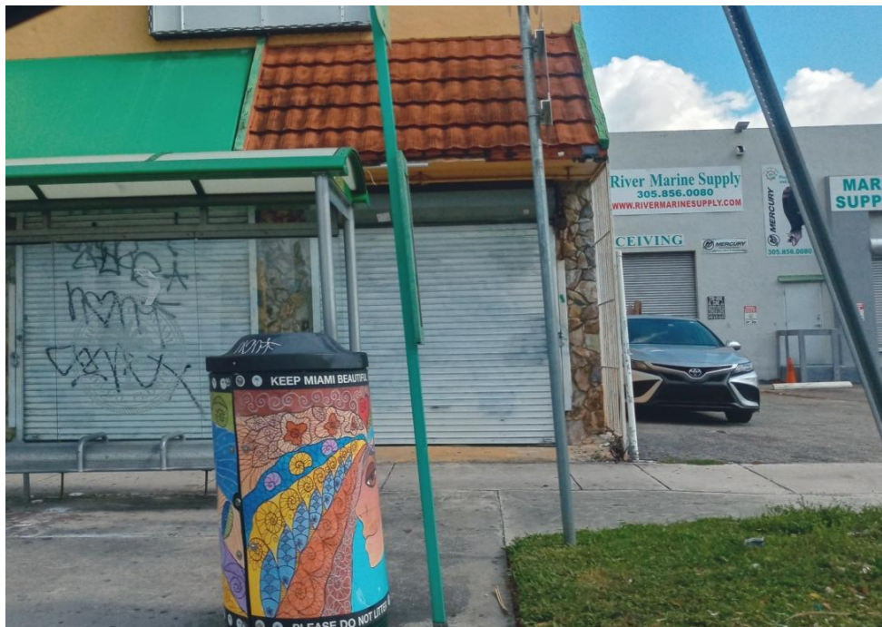
Exhibit: This photo illustrates evidence of site deterioration and inadequate transit stop. These defective conditions contribute to disinvestment.
